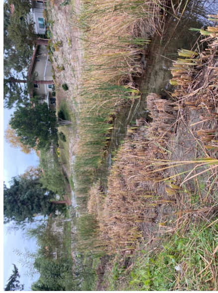
Photograph 6b After. Cut and chemically-treated cattails. Improvement in water visibility and flow immediately observed.
