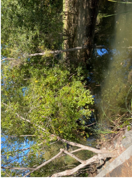
Photograph 5a Before. Taken south of the pedestrian bridge. Willow tree limbs encroaching into creek and partially obstructing flow.
